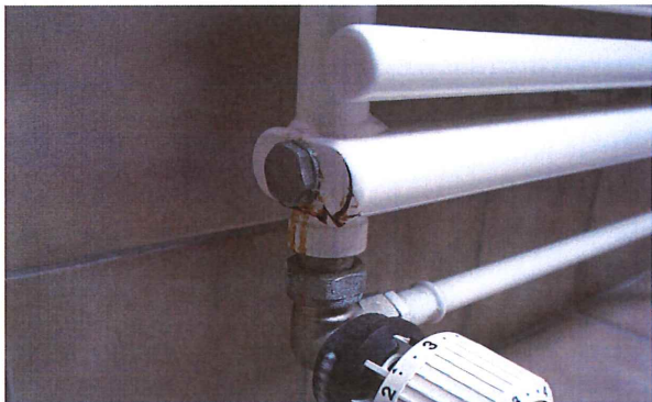
Handtuchradiator Bad DG
